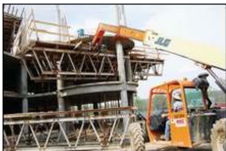
Workers at the Braxton Condominiums remove a table out from under the 3rd floor after the concrete has dried. MATT ANDERSON/THE TIMES
